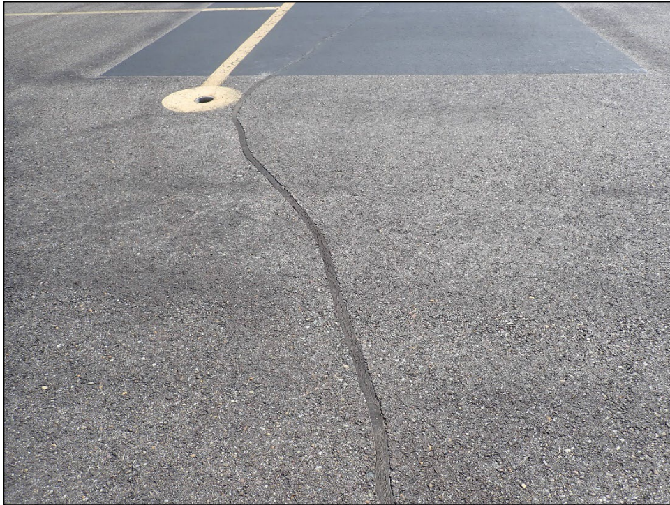
AP-11-14: L&T Cracking
