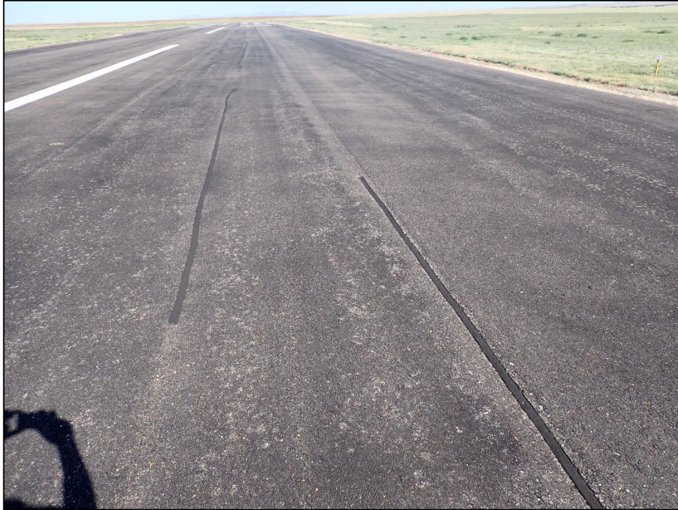
RW05-11-10: L&T Cracking
